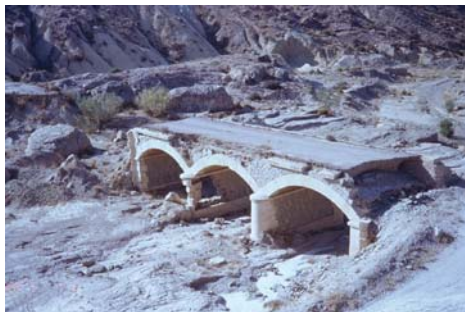
Damage caused by a flood.
