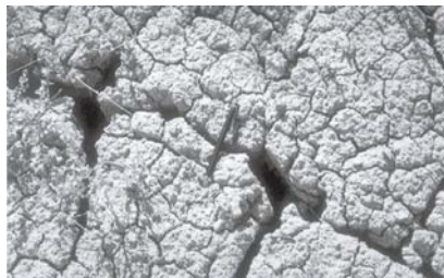
Fissures and cracks in the surface.
